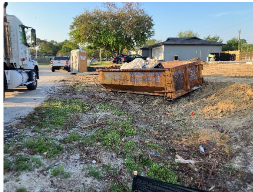
Figure 2 - Swale is being blocked by dumpster and missing temporary culvert pipe.
