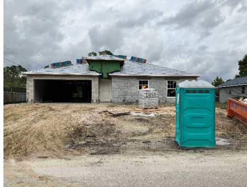
Figure 3 - No temporary culvert installed, porta potty and dumpster in the swale.
