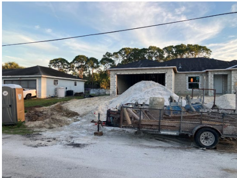
Figure 1- Swale is being blocked from a pile of dirt and porta potty, also is missing temporary culvert pipe.
